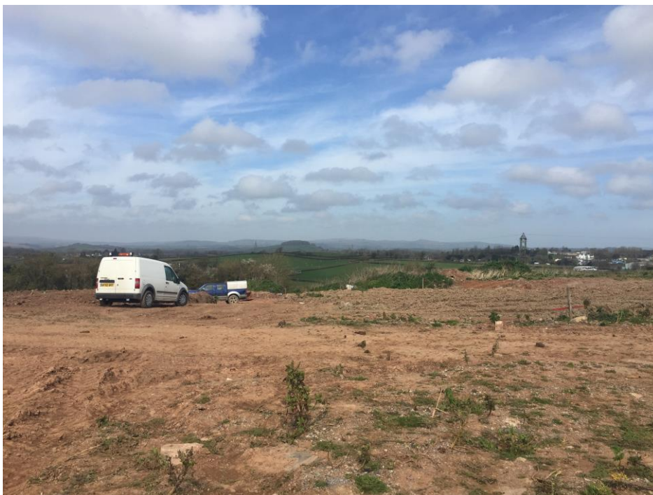
Looking north-west over Phase 5 – this is currently where the site is being regraded
