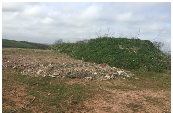
Top soil stores in the centre of the site with the material in Phase 2 still requiring regrading into the existing levels
